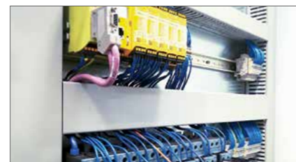
Main cabinet – safety PLC and Profibus
