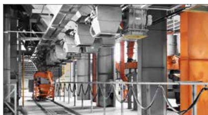
Refractory plant: dosing and weighing section
