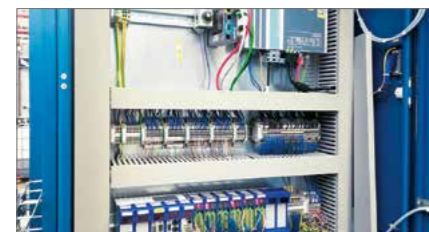
Bus box with box pc, axes controller and Profinet
